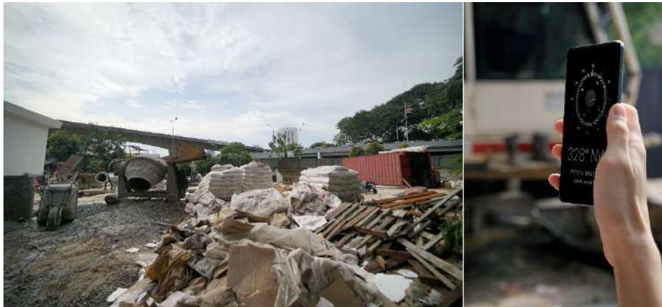
Fig.4. On left, photograph of site under renovation, On right, digital compass to measure the location and orientation
